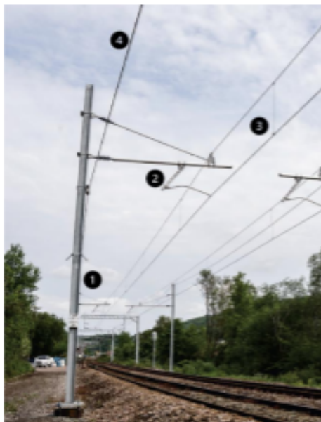
Example of Overhead Line Equipment:
